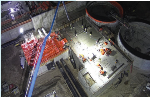
Blower Building and Gravity Thickeners
