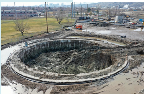
Influent Pump Station
